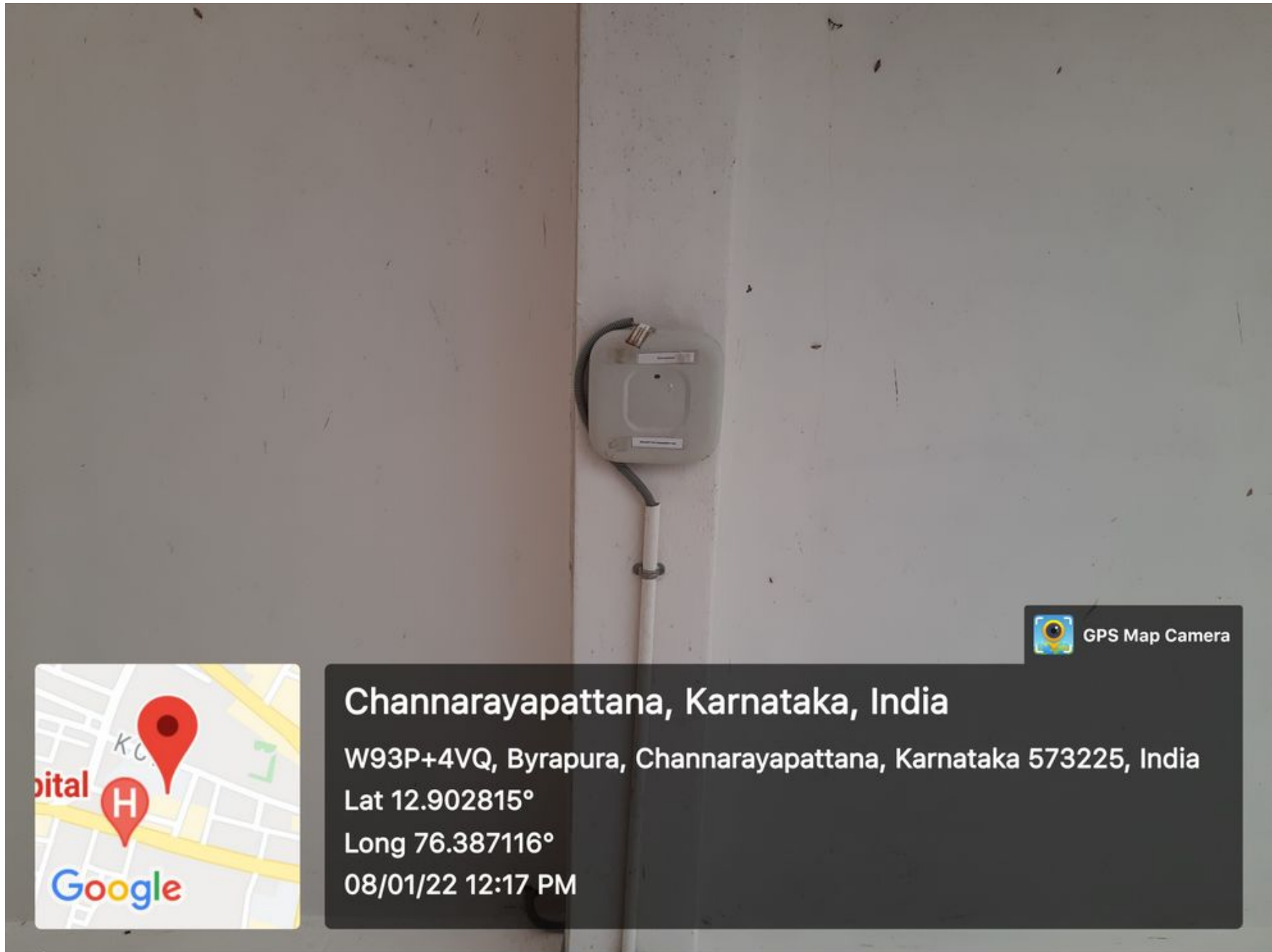
Router in Ground
